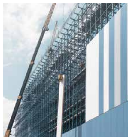
Special coating for use in maritime environments: Deep-freeze high-bay storage in warehouse in Grimbsby
